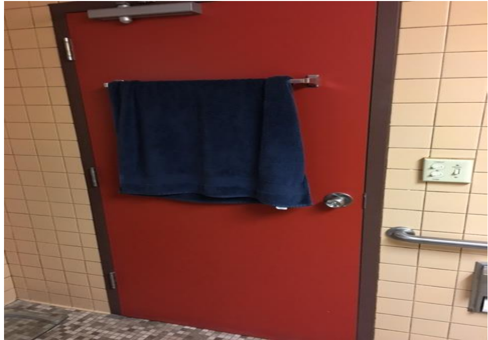
Photograph 7: View of lead containing red door/ brown door frame within the Captain's restroom.
