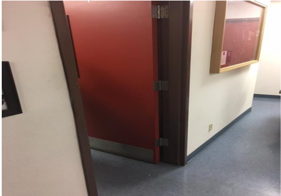
Photograph 3: View of representative lead containing red door and brown door frame.
