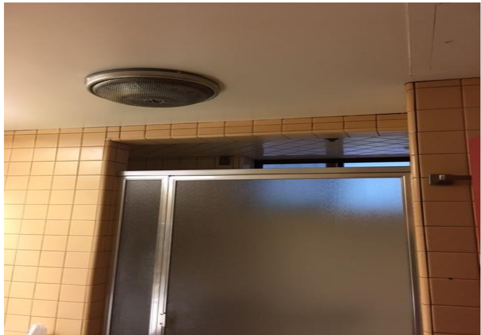
Photograph 8: View of lead containing black window frame within the Captain's restroom.
