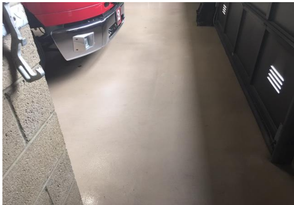
Photograph 6: View of lead containing gray flooring within Apparatus area.
