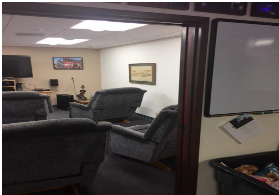
Photograph 4: View of lead containing sliding brown door and brown door frame.
